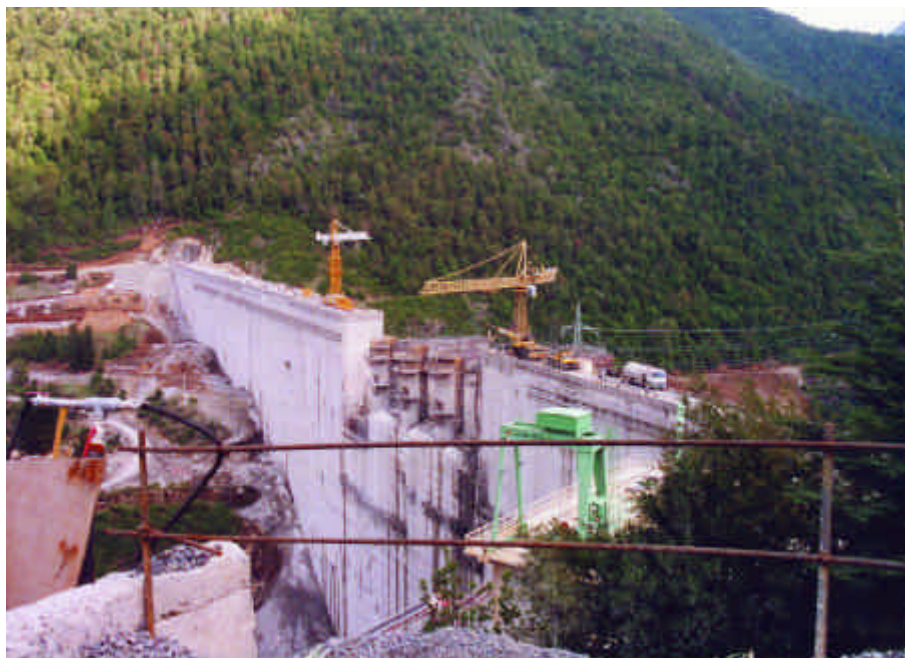
Chile led Latin America in deregulating and privatizing its electricity sector. Privatized utility Empresa Nacional de Electricidad S.A. (Endesa), which became Chile’s largest private company, developed or acquired hydro projects in Chile and elsewhere in Latin America through the 1990s, including the 450-mw Pangué Hydroelectric Project on the Biobío River, shown above near the end of construction in 1996.
